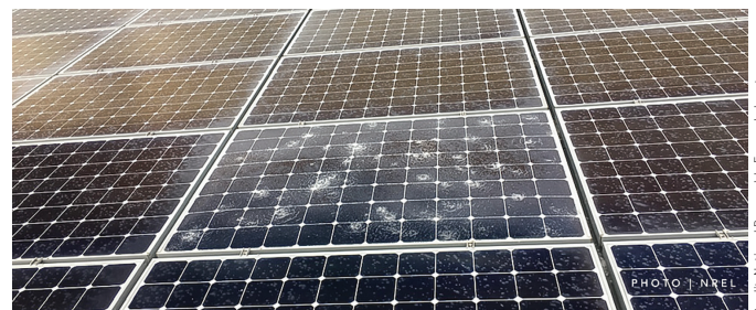
A solar panel that sustained damage during a hailstorm. If solar energy is to be a reliable source of energy, the resistance of photovoltaic modules to hail damage must be improved.
