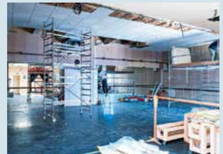
Saint-Gobain glass wool provides sound insulation at the Mogador Theatre in Paris.
